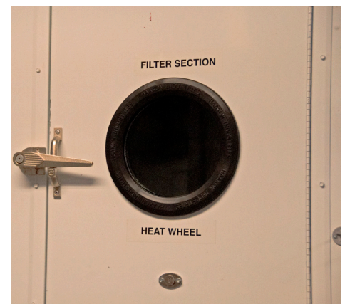
The heat wheel takes the warm moist air that we're exhausting from the building and preheats the incoming cold air as an energy-saving feature.
