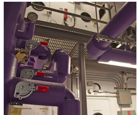
The main air handling unit is two-stories high: Air leaves through the top section of the unit. On the inside, the heat wheel spins and preheats air in the bottom section of the unit.
